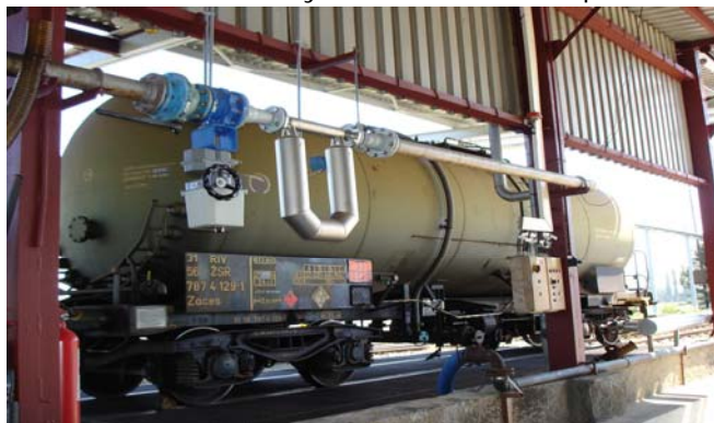
Pumping solvents from a railway tank
