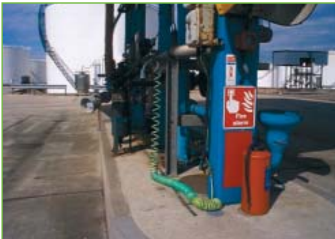
Figure 1. Typical bottom loading stand with earth connection
